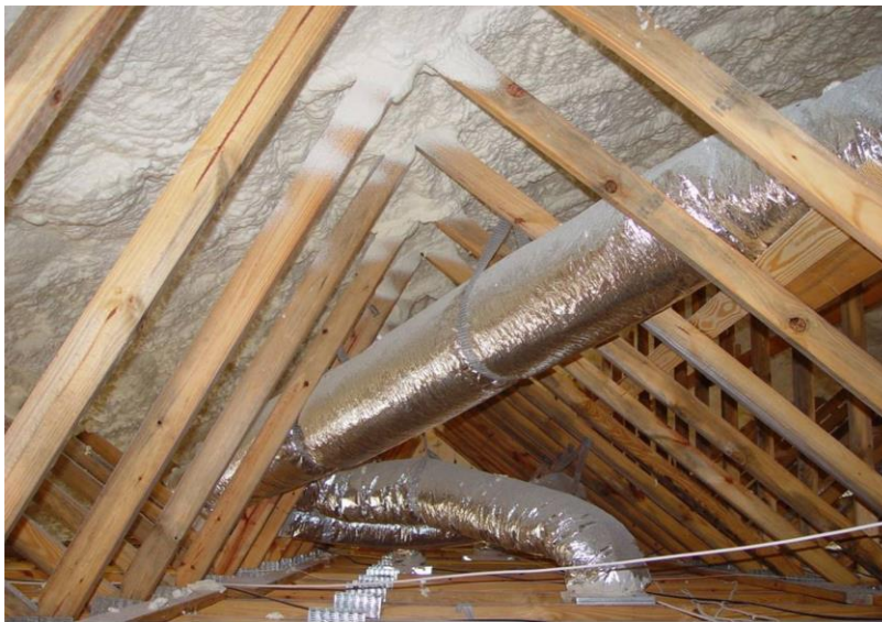
Figure 2 - Actual installation of SPF in an unvented attic. Notice that ductwork is now in conditioned space.
