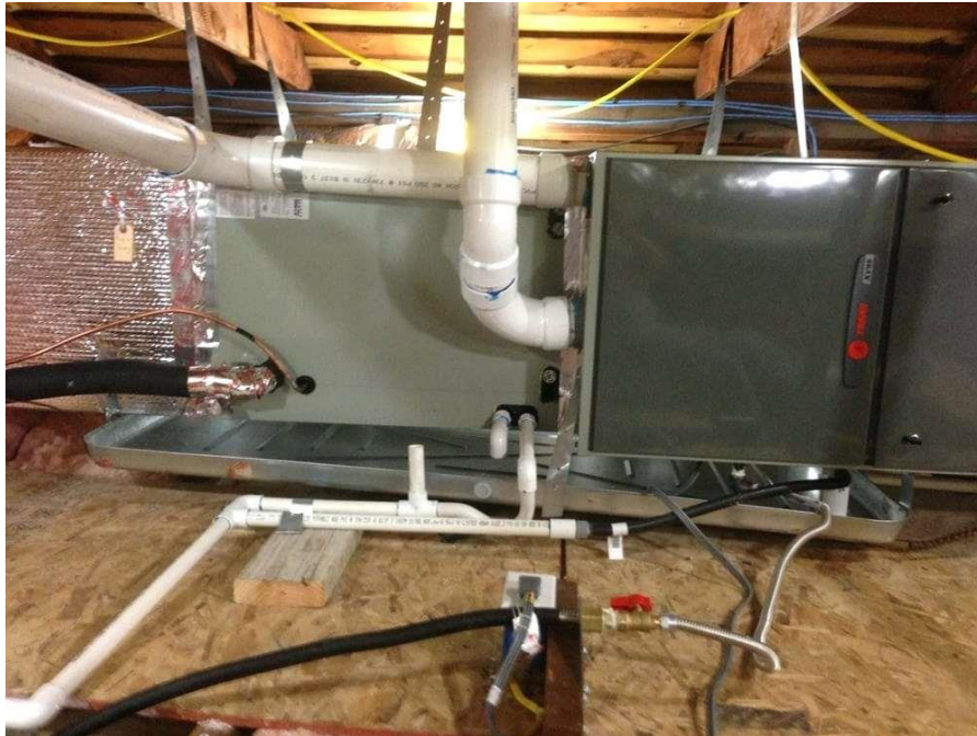
Figure 4 - High-efficiency gas furnace in an attic space. Note large-diameter PVC pipes used for combustion air and exhaust gases.
