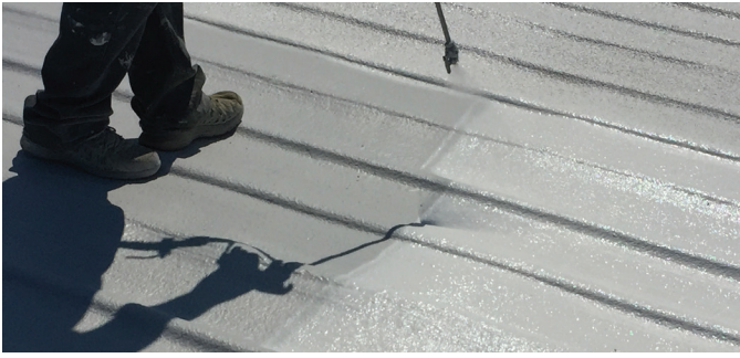
Application of SPF over a metal roof followed by an acrylic coating.
