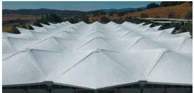
SPF installed over an unusual roof design at Birkenstock headquarters in Novato, CA.
